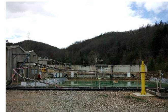
Water treatment plant in Bertholène
